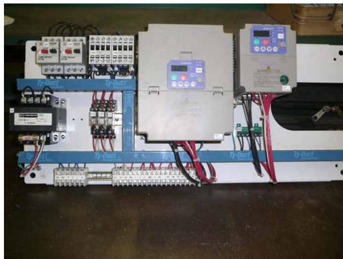
Hitachi's SJ200 Series integrated on Detroit Hoist standard hoist design
